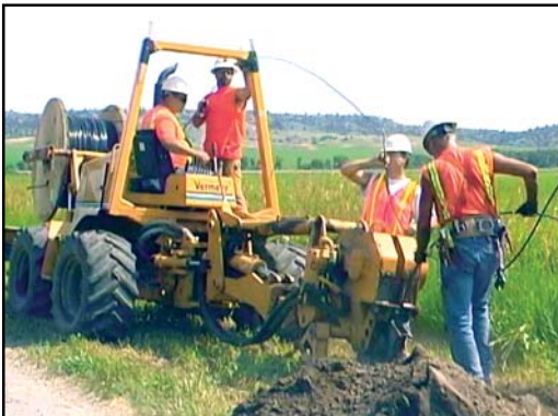
Crews of Nemont, the first telco to lay fiber in Montana, continue to provide high quality service to rural customers.
